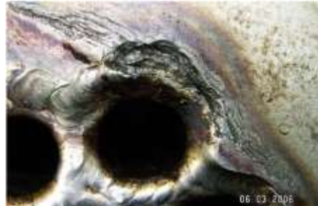
Figure 2: Crevice corrosion in seawater cooler (Wraglen p.179)
