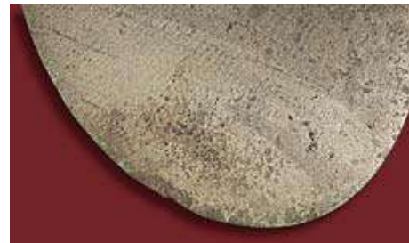
Figure 4. The pitted area closed to the blade tip is caused by cavitation
